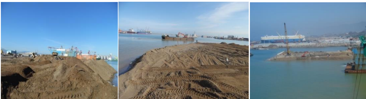
Figure IV. 1: Photos of the steps of backfilling of the caisson fabrication workshop Djen-Djen port Jijel-Algeria [57].
