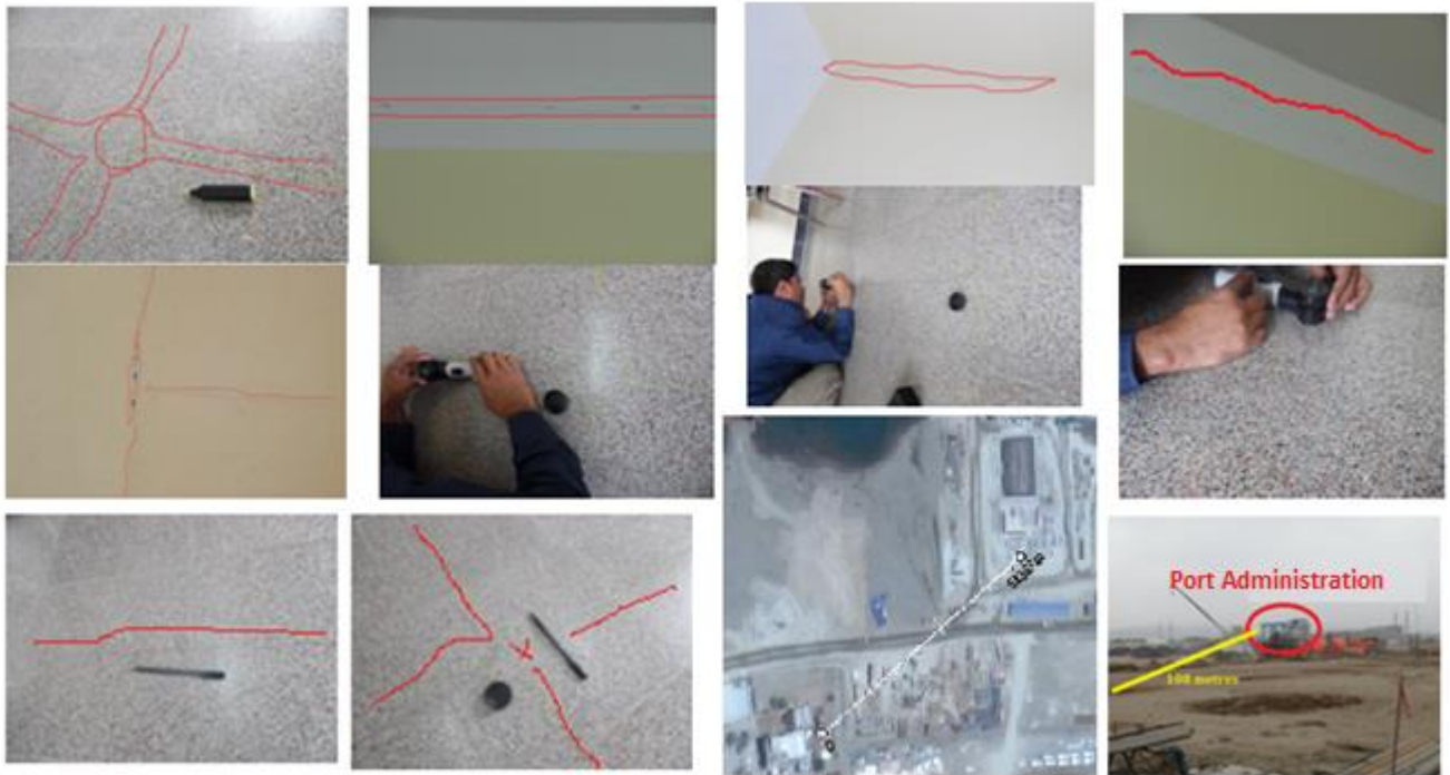
Figure IV.10: (a) Photographs of cracks in the port authority resulting from DC [57].
